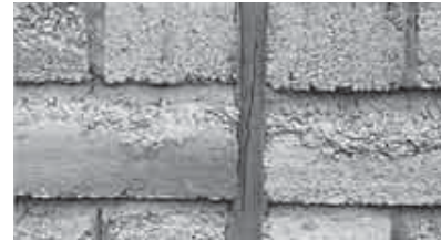
FIGURE 3.7 - SEALANT COHESIVE TEARING
