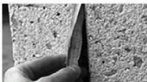
FIGURE 3.6b - SEALANT ADHESIVE BOND LOSS
