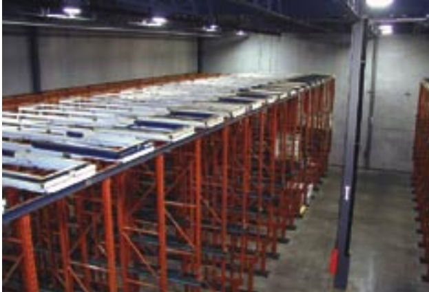
Push-Back Racking Above Drive-In Installation
