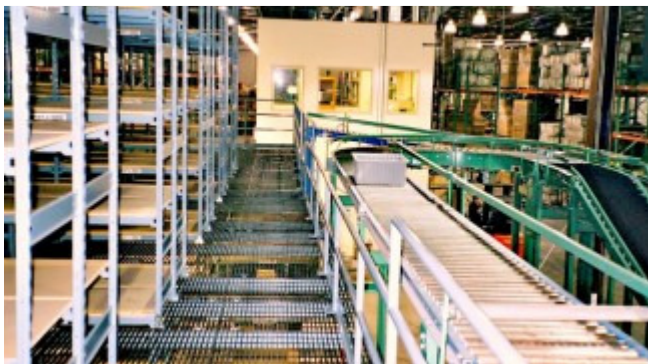
Integrated Conveyor on top floor of Multi-Level System
